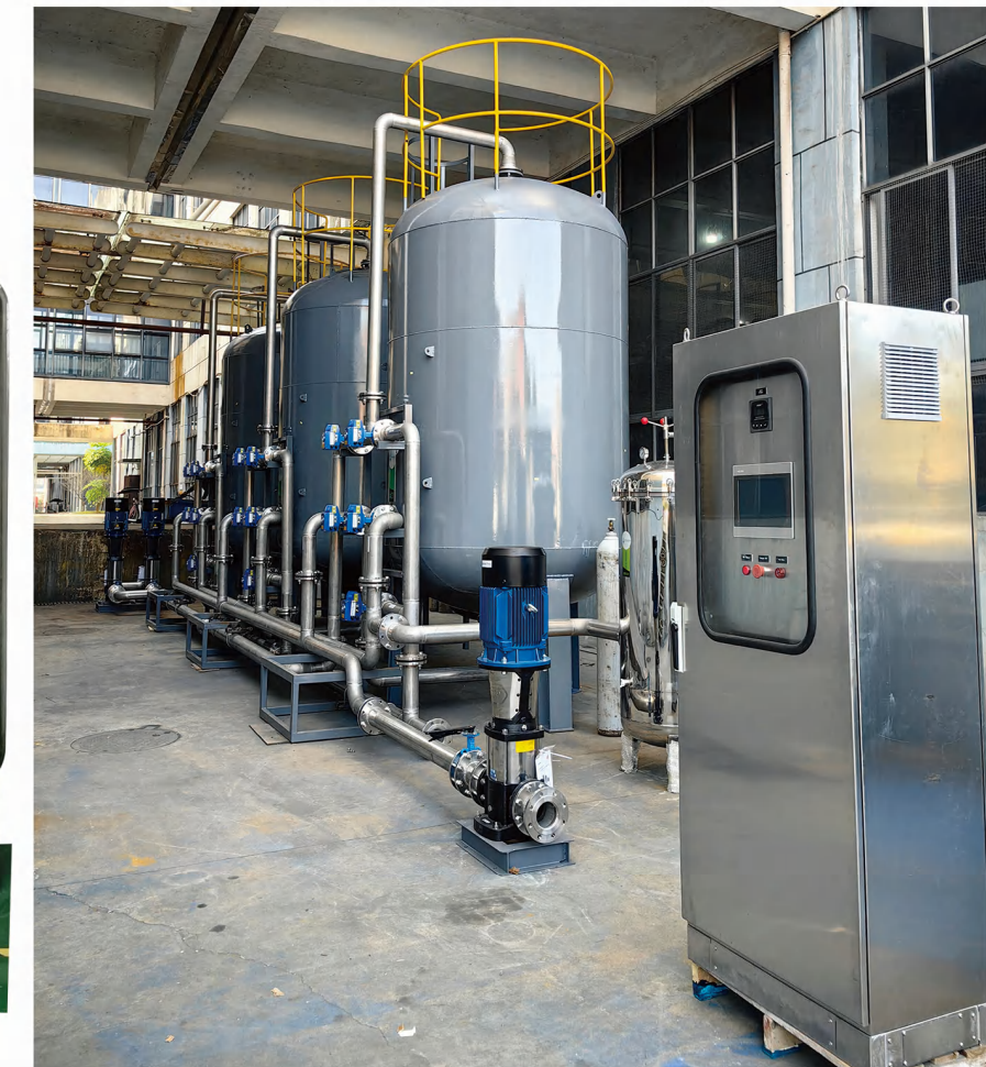
2000m3/Day Multimedia Filtration System Project
